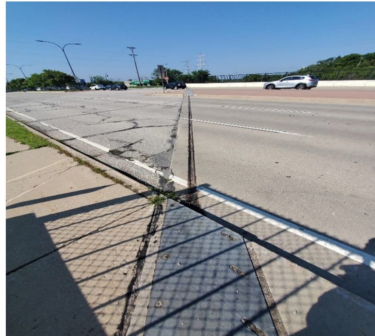
Expansion joint damage / leaks
