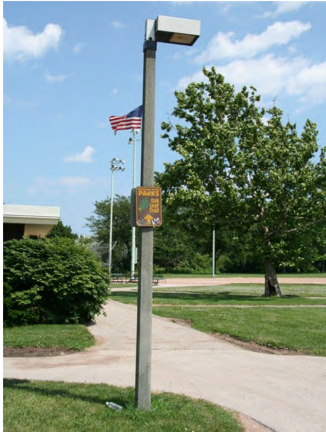
Box lighting found along pedestrian paths within Pulaski Park.
