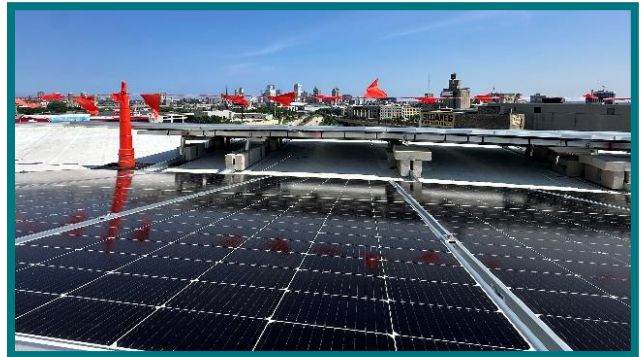
Rooftop solar panels at the Coggs building
