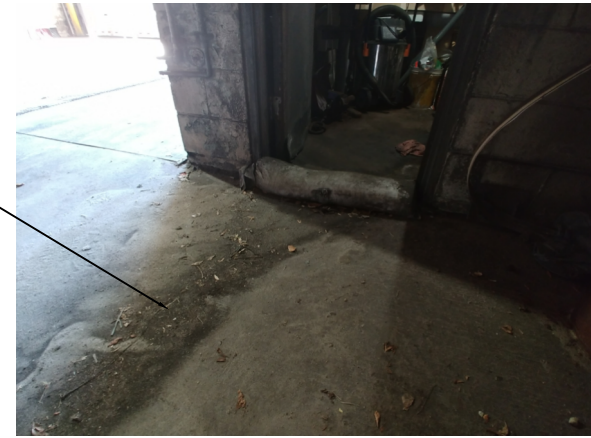
CLOSER VIEW OF FLOOR SLAB AREA IN FRONT OF DOOR TO EXISTING RESTROOM
