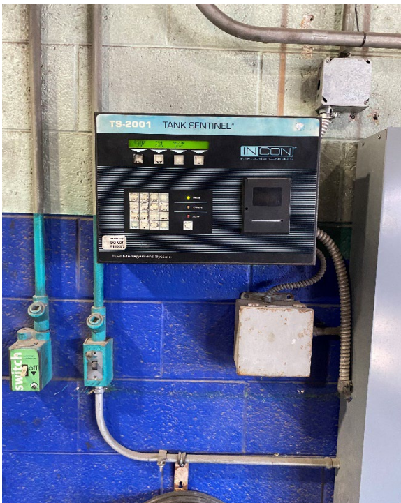
Figure 3: Maintenance Building (South Side) Automatic Tank Gauge (ATG)
