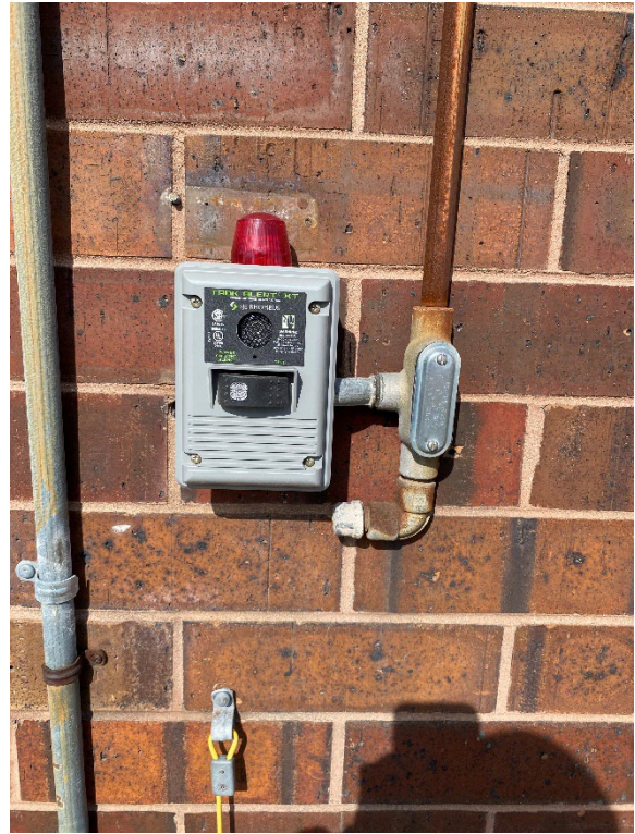
Figure 2: Maintenance Building (South Side) Overfill Alarm
