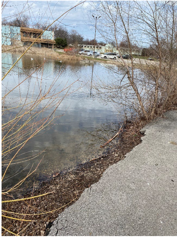
Figure 2: Picture of trail falling apart next to the lagoon.
