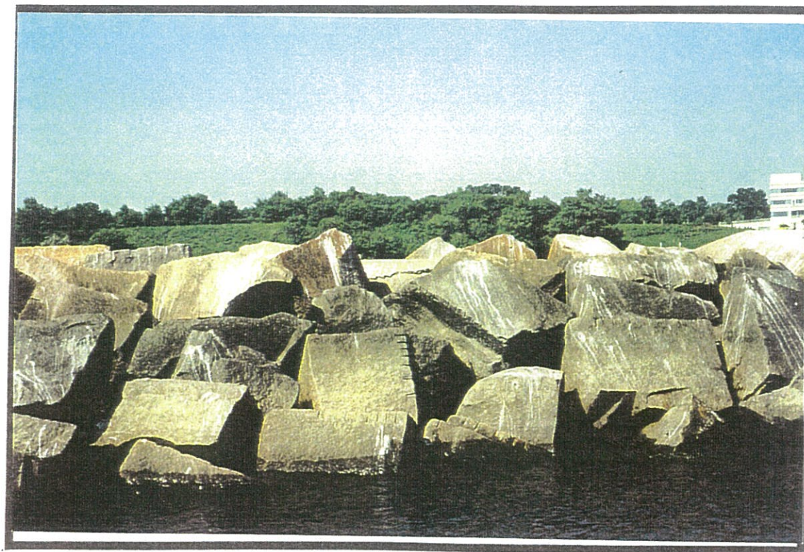
PHOTO #8: TYPICAL "GOOD" SECTION OF BREAKWATER. NOTE INTERLOCKING/ CHINKING OF STONE, ESTIMATED SIZE OF 7 TO 12 TONS.
