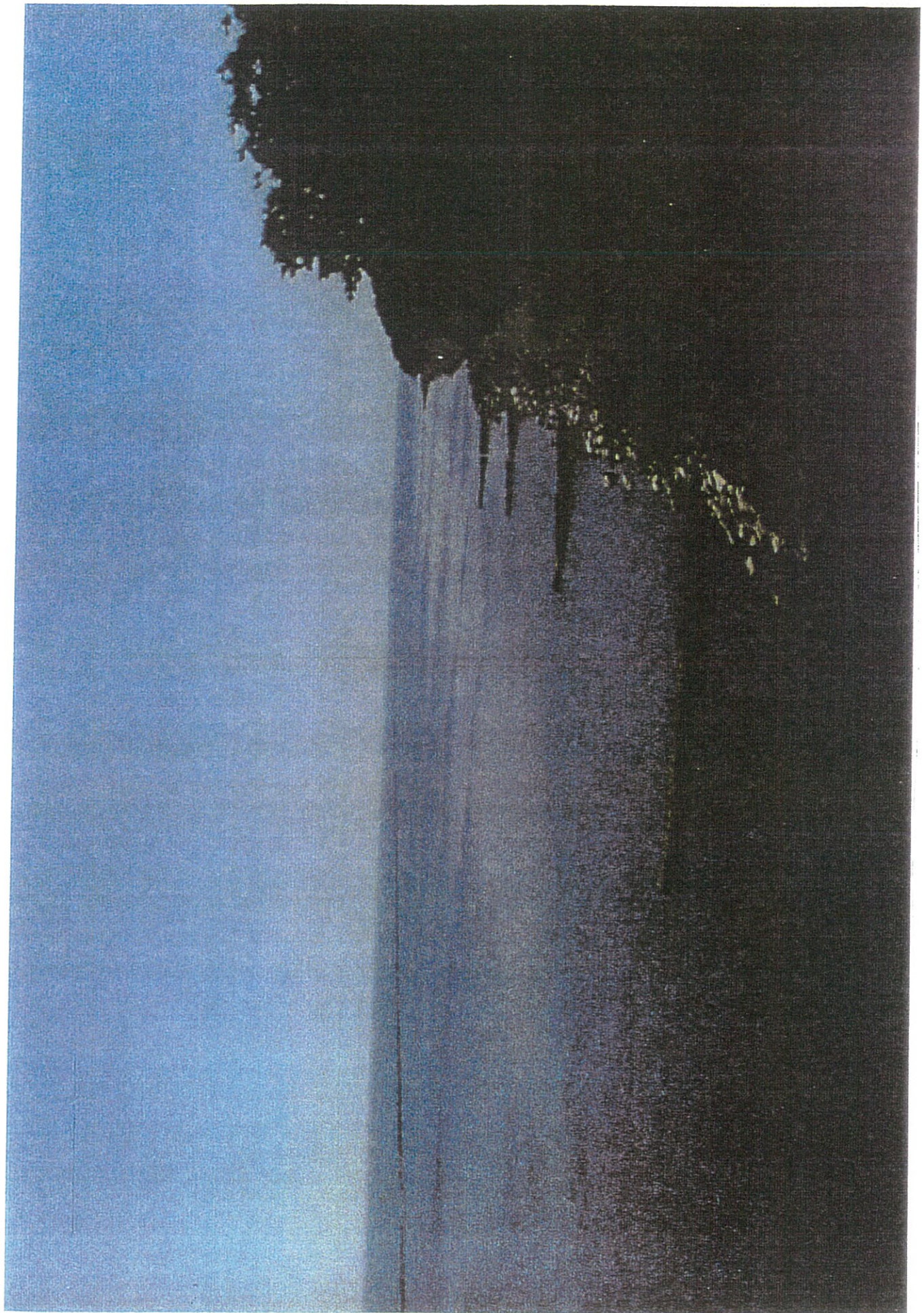
PHOTO #14: VIEW OF GROINS IN NORTHERN PROJECT AREA. NOTE DETERIORATION OF BREAKWATER.
