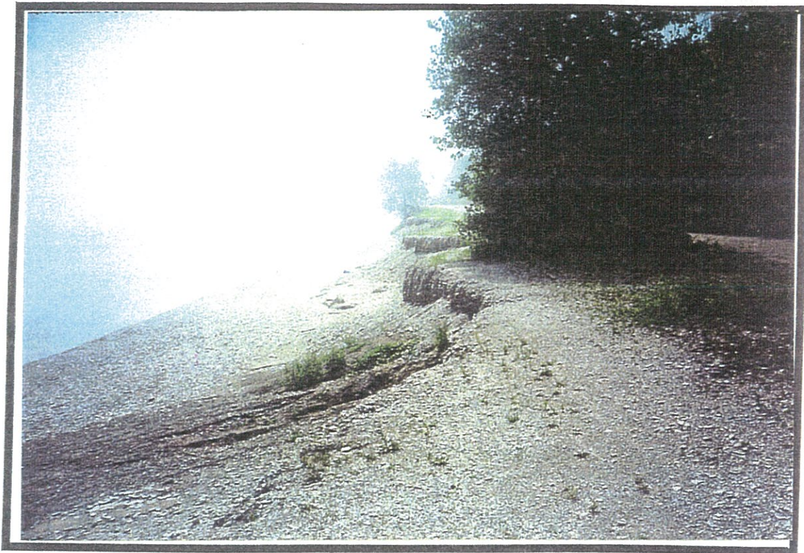
PHOTO #3: SHORELINE COVERED WITH SMALL STONE HAS ERODED
