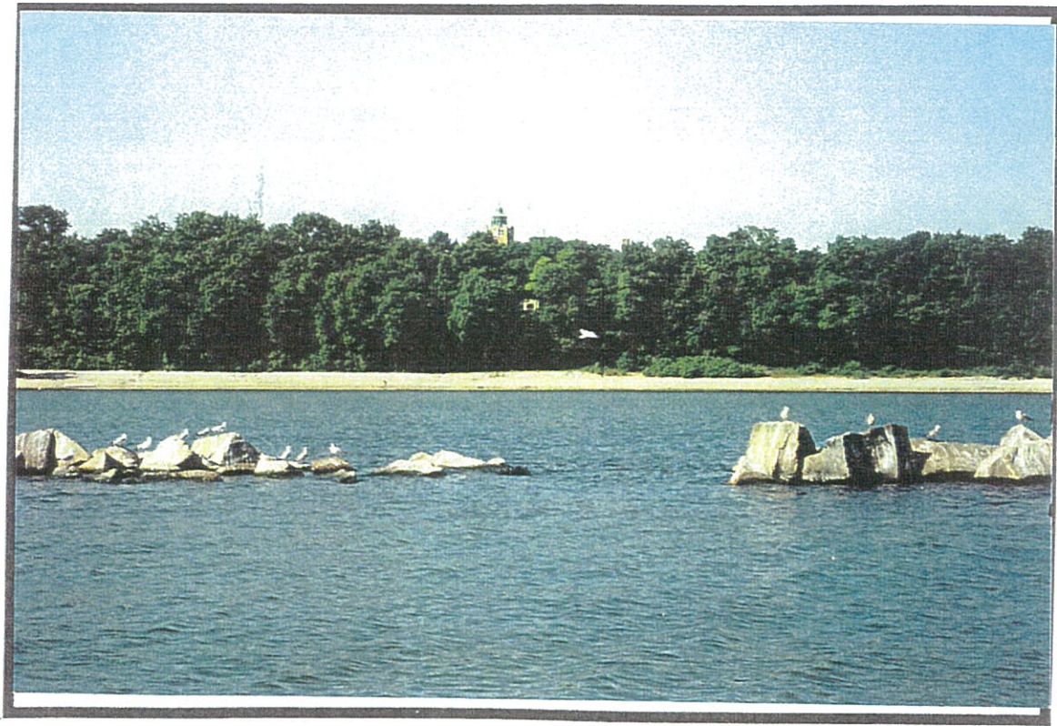
PHOTO #10: HOLE OR VOID IN BREAKWATER
