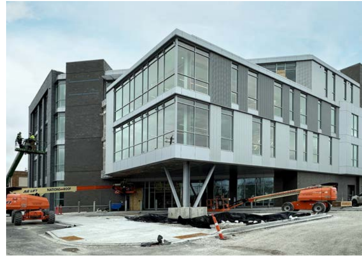
The new Marcia P. Coggs Health and Human Services Center under construction in 2024. It will be a four-story, 60,000 square foot building with the first floor intended to be a warm, welcoming, and accessible entry point for information, access to services, and community space.
