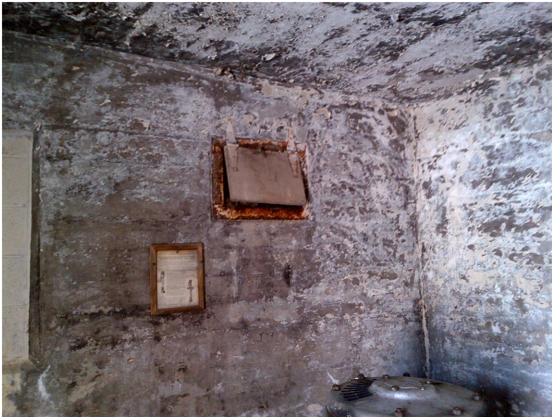
PHOTOGRAPH NO. 4: Subject Property – east wall – exhaust fan
